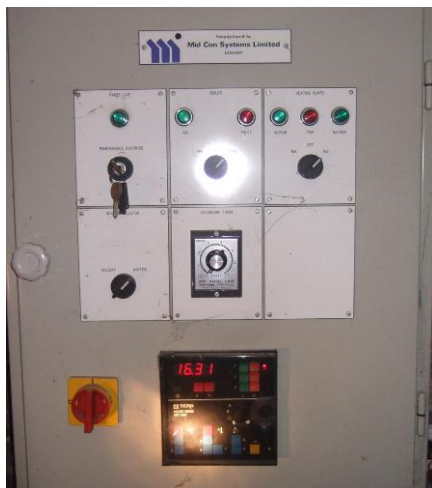
The boiler and heating control panel at Grasby All Saints
